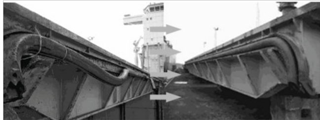
Damaged EVA - Seal Replaced by Gemlas Sliding Seal.
